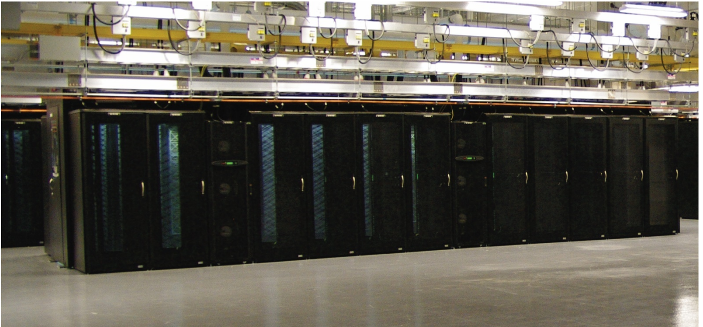
FIGURE 4. In-row cooling at the Massachusetts Green High Performance Computing Center (MGHPCC)
