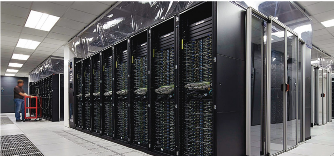
FIGURE 3. Hot-aisle containment inside BP's state-of-the-art Center for High-Performance Computing (CHPC) in Houston
