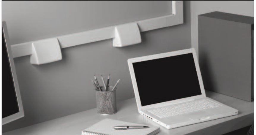
2400 Series Raceway shown with our new Downward Facing Receptacles in a typical school library application.
